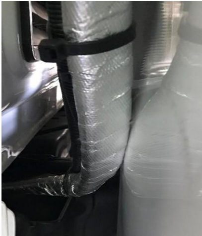
Figure 1.20: Hose Rub (NOT ACCEPTABLE)
