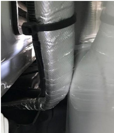
Figure 1.20: Hose Rub (NOT ACCEPTABLE)
