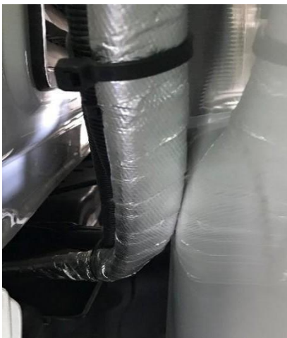
Figure 1.22: Hose Rub (NOT ACCEPTABLE)
