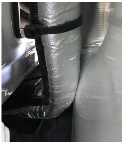
Figure 1.19: Hose Rub (NOT ACCEPTABLE)
