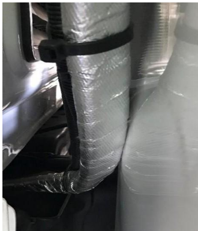
Figure 1.20: Hose Rub (NOT ACCEPTABLE)
