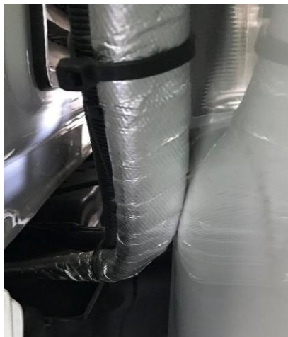
Figure 1.19: Hose Rub (NOT ACCEPTABLE)
